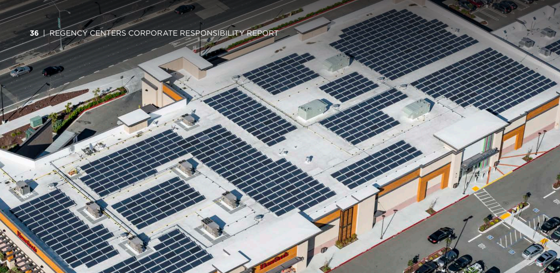
Persimmon Place | San Francisco, CA | Rooftop Solar Photovoltaic System
