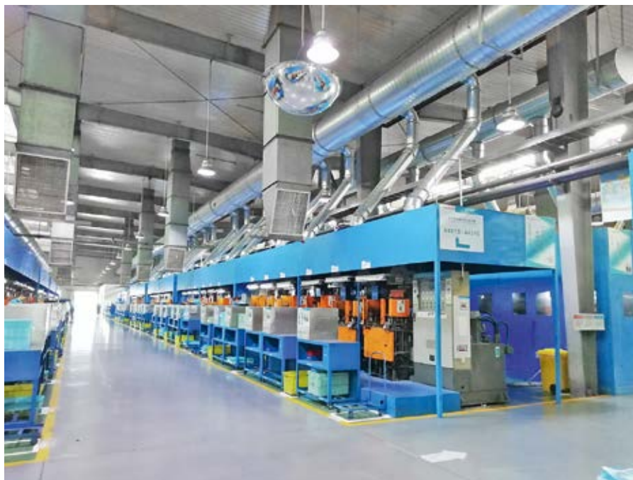
The new exhaust air purification systems at the Chinese plant improve air quality.
