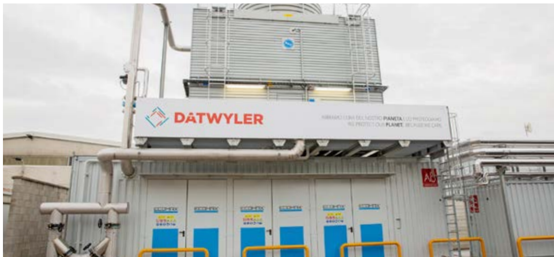
The Italian plant commissioned a combined heat and power plant in 2019 to ensure a more efficient supply of electricity and heat. Thanks to the new environmentally friendly heating/cooling method, Datwyler is reducing CO 2 emissions by 900 tonnes per year.
